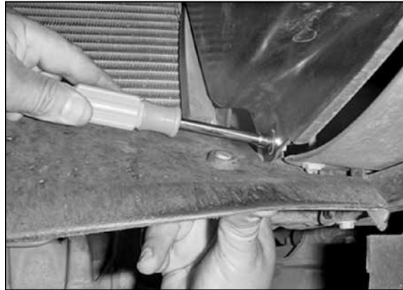
31. Loosen and remove the two bolts that retain the lower radiator cover to its mounting brackets.
